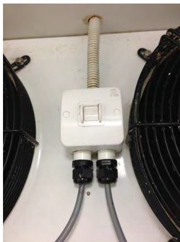
Fig.23 The fan switch in the cool room
