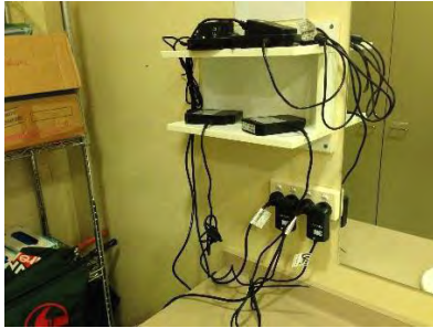
Fig.7 PAPR battery charging station
