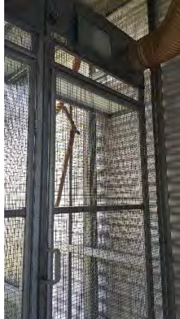
Figure 5: Outdoor access slide open (all cages)
